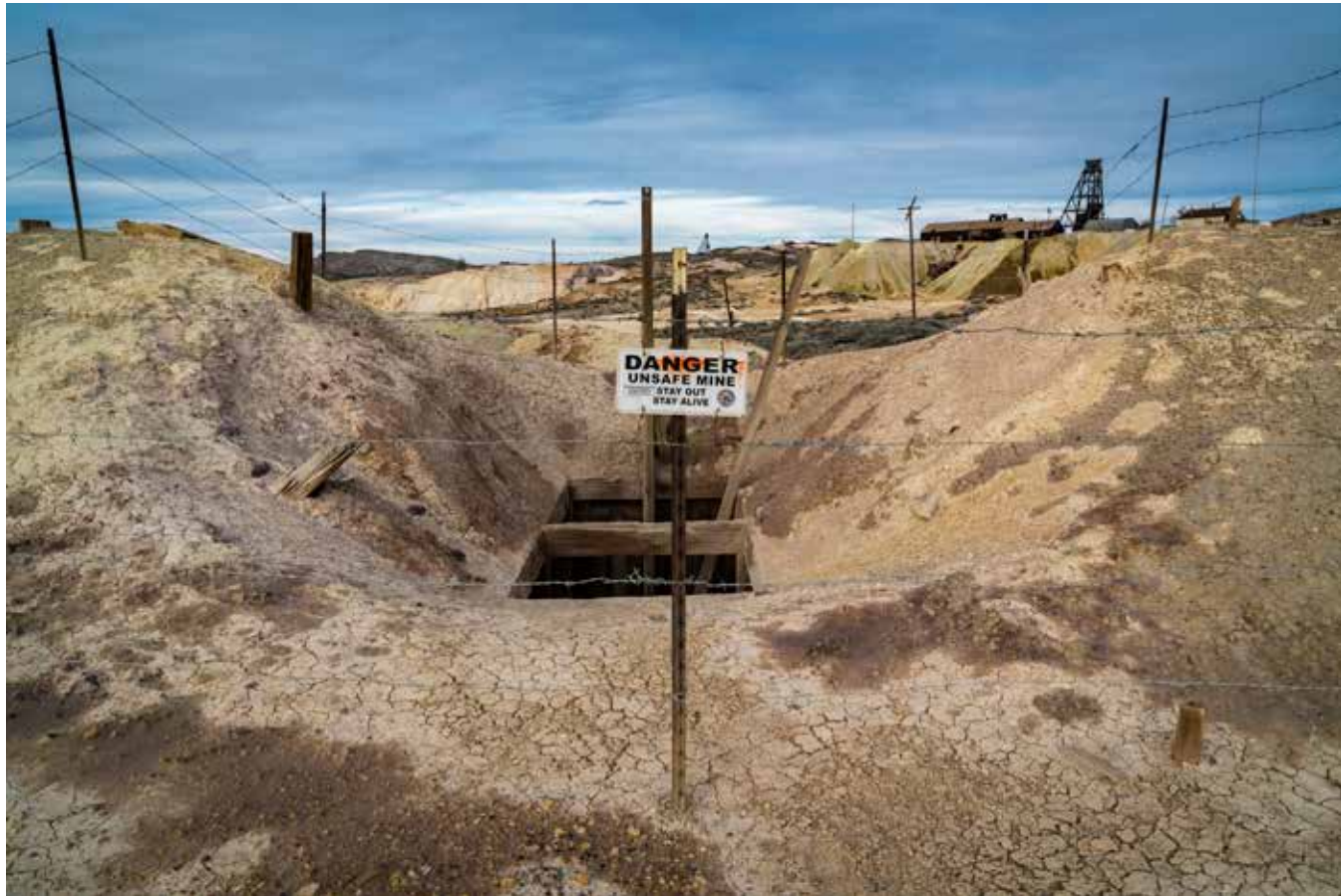
Thousands of abandoned mining hazards like this one in Goldfield's historic mining district are scattered across the Mojave Desert.
